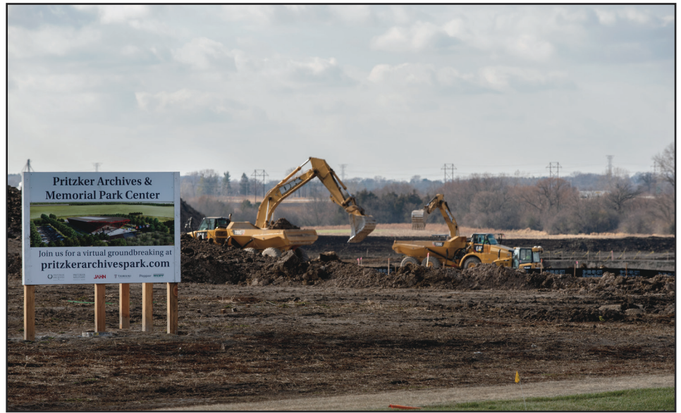
Heavy equipment grades the site of the Pritzker Archives and Memorial Park Center.
