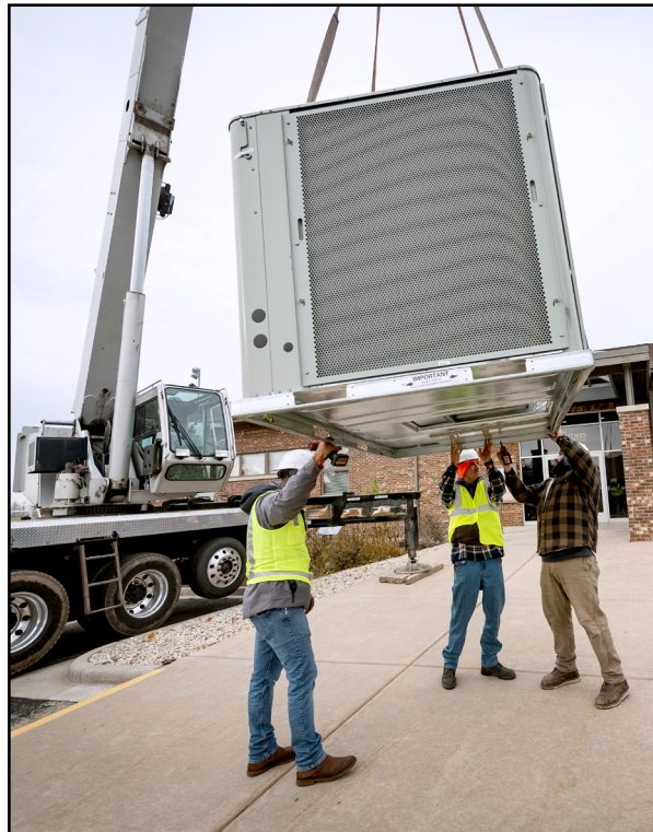
Kenosha Heating and Cooling employees use a crane to lift a new HVAC unit to the roof of the Village/Town Hall.
