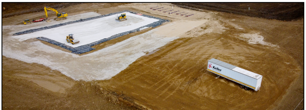
Grading is ongoing at the site of the proposed service center at Highway E and East Frontage Road.
